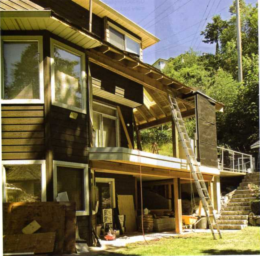
West Vancouver dream backyard in progress. Pool, barbeque & patio retreat. Photo courtesy of RJR Construction.
